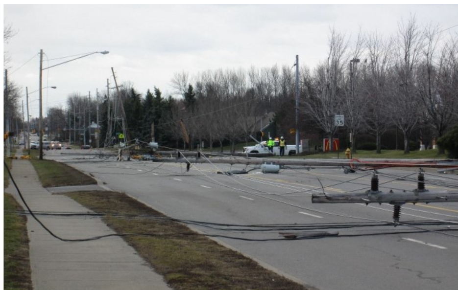
A severe wind storm in early March 2017 downed distribution lines in Rochester, N.Y. | New York PSC
